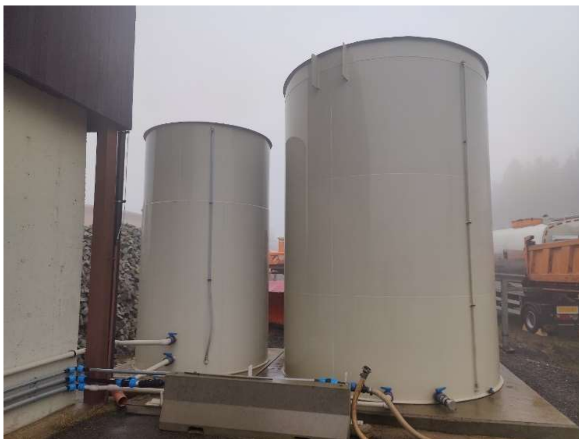
Figure 4 – Tanks for magnesium chloride in the road administrator's facility Bystřice n/P
