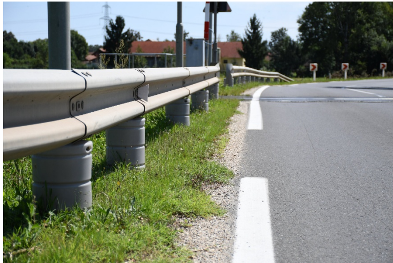
Figure 3.18 : Protective shock-absorbing elements mounted around the support posts of the SSB
