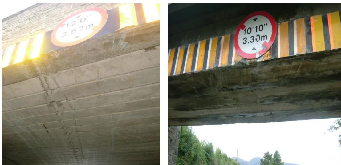
Figure 4.1: Bridge warning signs and damage to concrete under the bridge (Byrne, 2009).
