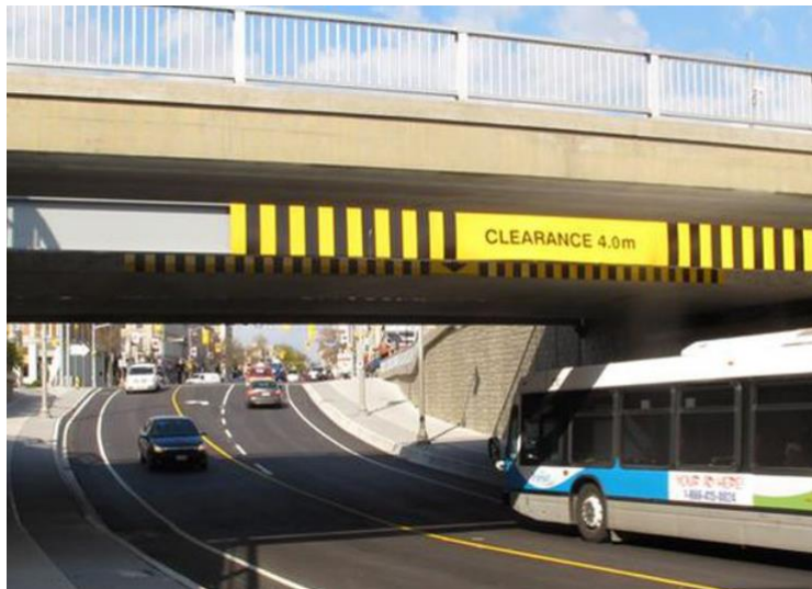
Figure 4.2: Crash beam for preventing bridge strikes (Guelphmercury, 2021).
