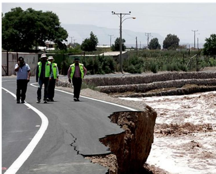
Fig. 4 – Road Administration Agents checking road damages
