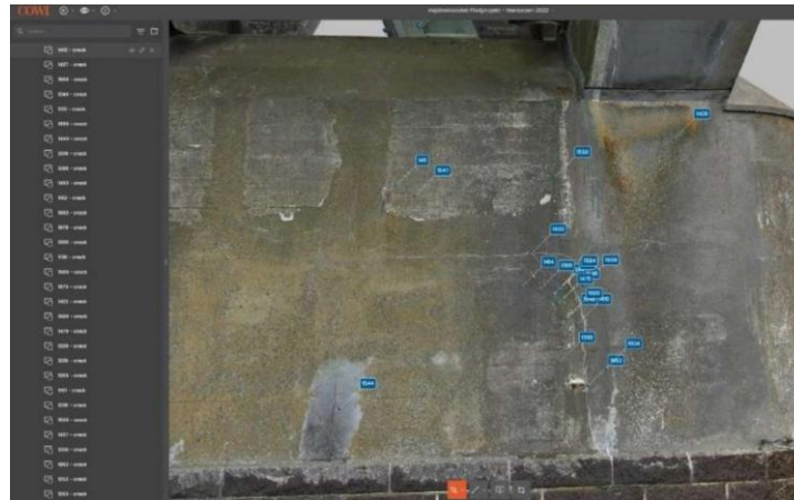
Figure 5.5: Example of AI annotation of cracks.
