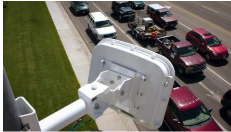
Figure B.25: Radar and infrared sensors monitor traffic, while AI analyses data for real-time insights, optimising road management and incident response (Wavetronix SmartSensor Matrix, 2024).
