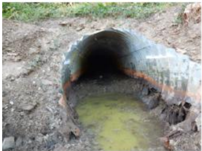
Figure 34. An example of poor maintenance of a culvert: sedimentation filled nearly half of the culvert volume (France, courtesy Cerema St. Brieuc)
