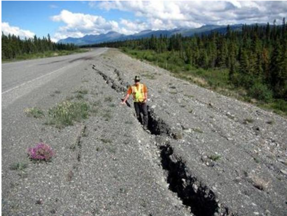
Figure 12. Effect of ice on an embankment (Canada)
