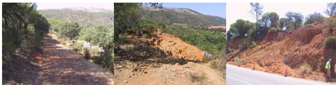
Figure 30. Various examples of events affecting earth structures. Top, flooding after heavy rainfall. Middle, fire and rockfall. Bottom, change in land use: as a result of the construction of new mountain tracks and firebreaks upslope, new runoff paths (not previewed in the initial design of the road) have been produced after rainy periods.
