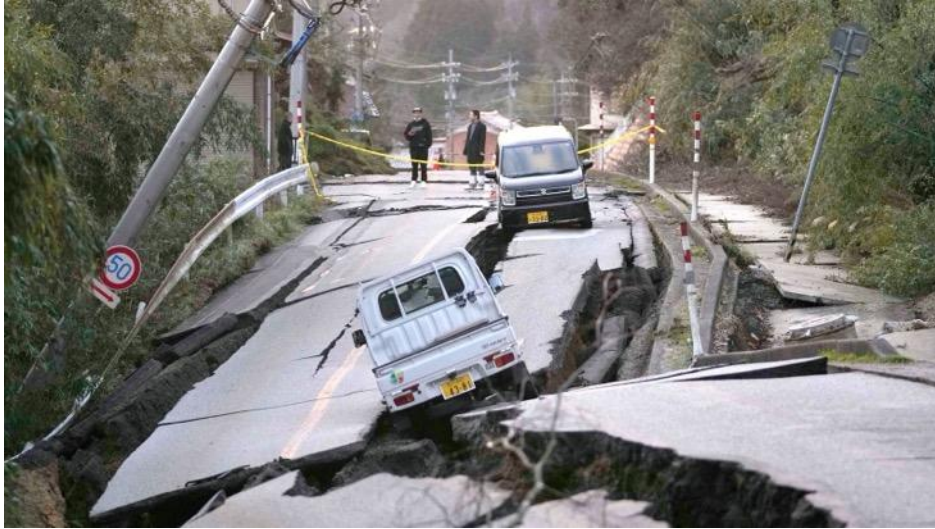
Figure 10. Effects of earthquake on a road (Japan)
