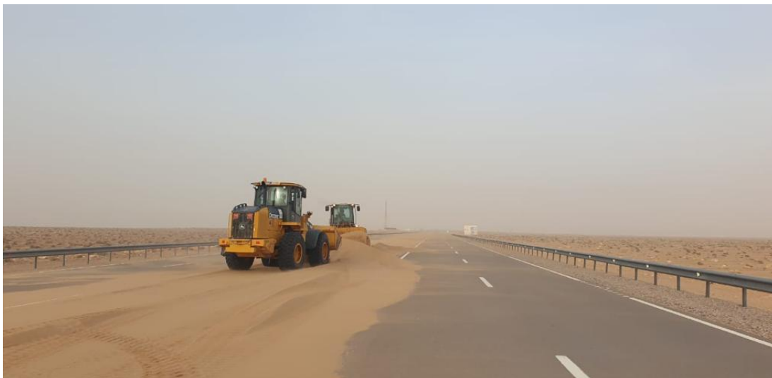
Figure 5. Effects of wind action on earth structures (Morocco)
