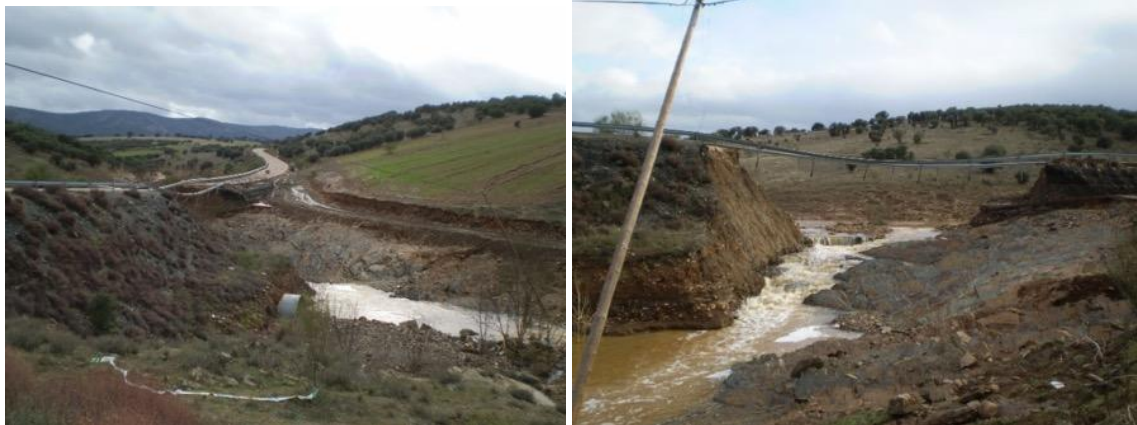
Damage of an embankment due to heavy runoff
