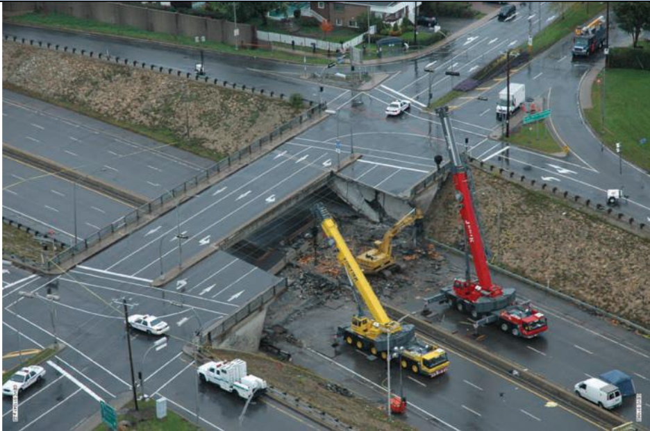
General view of the collapsed bridge
