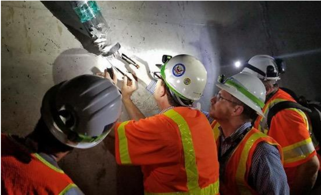
Figure 8: A group of engineers and scientists investigating the failure of a post-tensioning tendon.
