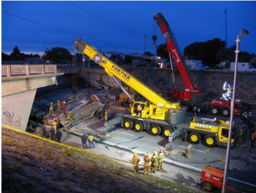
Figure 7: First responders investigating the site of the De la Concorde overpass collapse outside of Montreal, Quebec, Canada on September 30, 2006.
