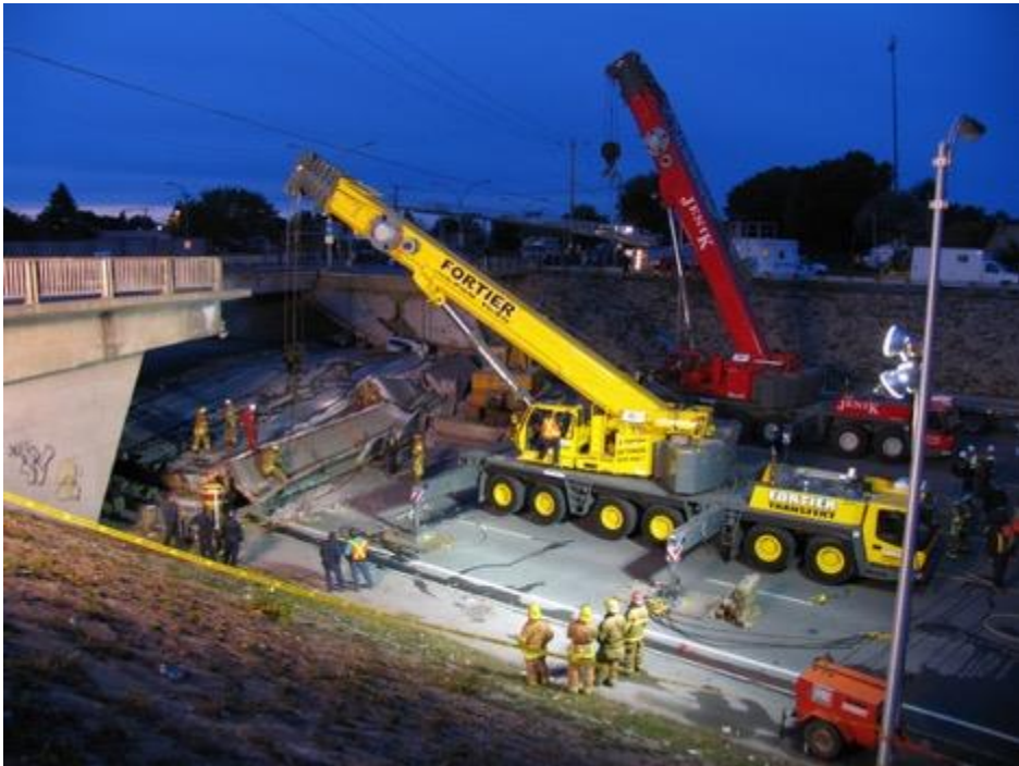
Rescue operations on the collapsed center span
