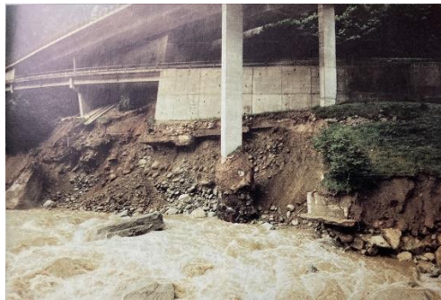
Picture 4: washed-out foundation Pillar J; In the foreground a washed-out framework foundation that remained there. In the background the washed-out foundation of the sustaining wall carrying the cantonal route.
