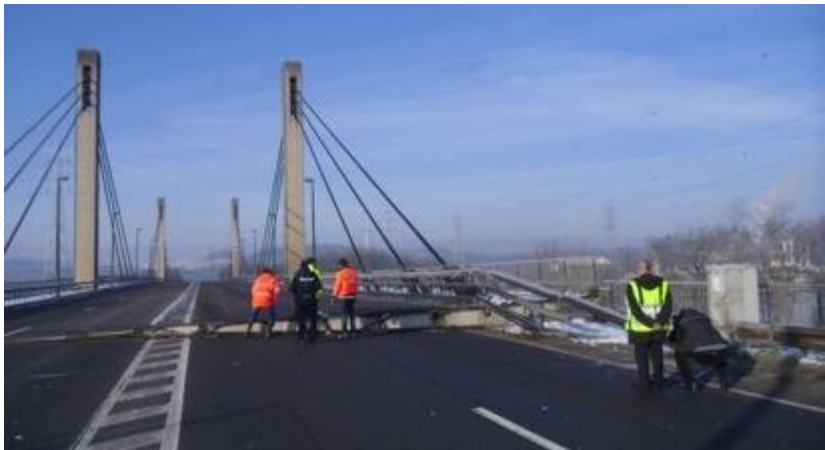
Picture of the support after failure
