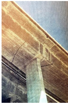
Picture 2: Girder Box cracked over Pillar J
