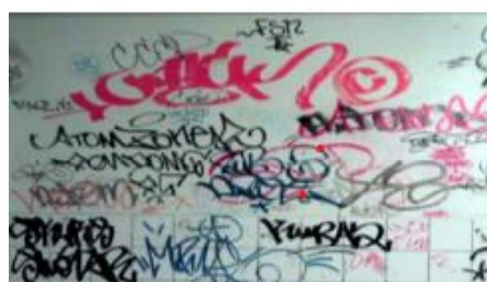
Graffiti that needs to be removed FEDRO photos
