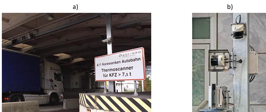
Figure 5.1 Thermo-scanner facilities to detect overheated heavy vehicles, Karawankentunnel, Austria; a) a truck entering the tunnel; b) thermal cameras installed at the tunnel's entrance; ©ASFINAG.
