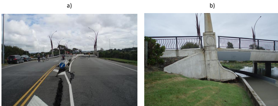
Figure 4.8 Damage to a bridge structure in Canterbury resulting from liquefaction in Christchurch earthquake. a) fissures and settlements on the bridge approach; b) an abutment rotation; ©NZTA.
