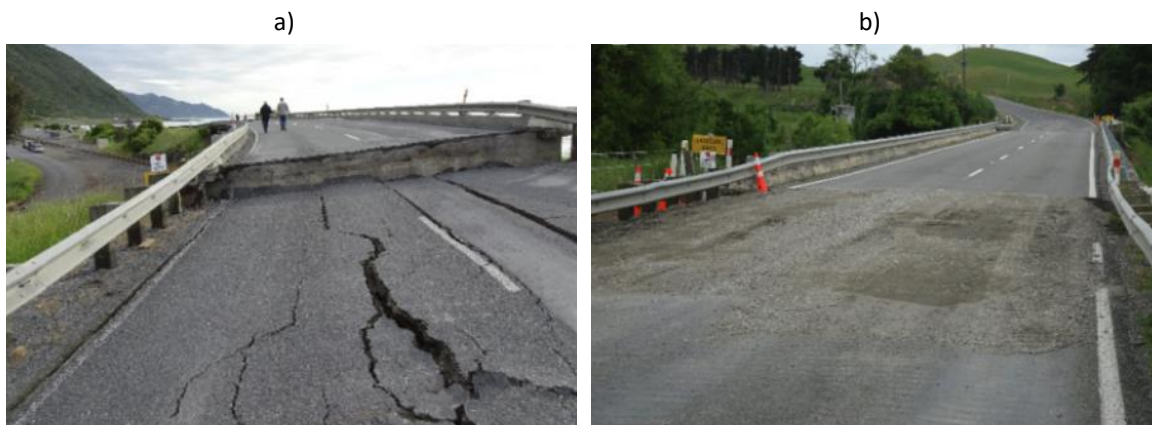
Figure 6.3 Settlements at bridge abutments in Kaikōura earthquake, New Zealand; a) a severe settlement (>0.5m) at a bridge near Oaro; b) a minor settlement mitigated with a temporary ramp (fill); [61].
