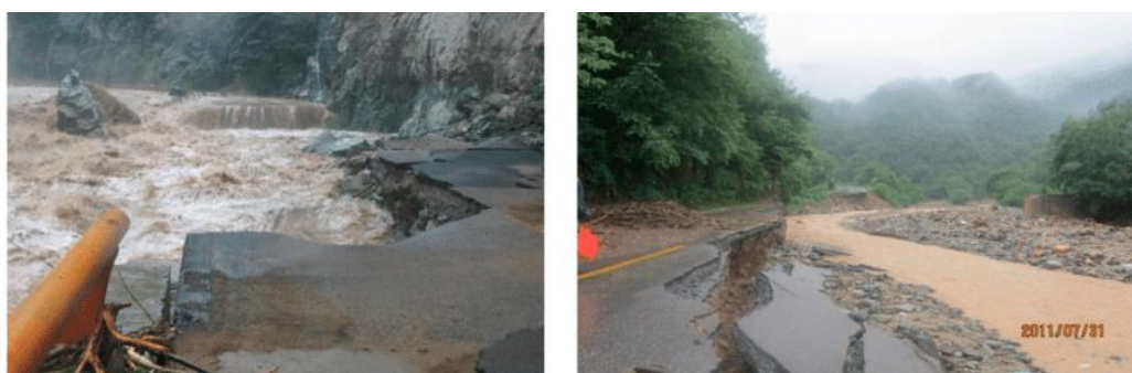
Figure 6.20 Whole width flood damage to highways in Shaanxi Province, China, [74].
