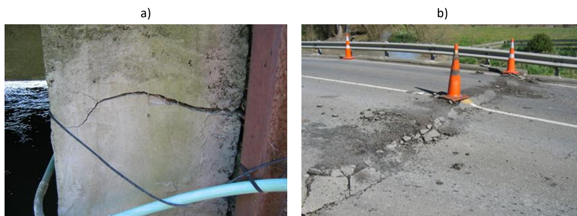
Figure 4.9 Various damage to a bridge in Canterbury in the Christchurch earthquake. a) cracking of a bridge abutment; b) settlement of an abutment; ©NZTA.
