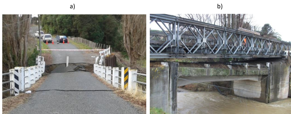
Figure 6.13 Response to a bridge failure due to scour, Arapata Road, Manawatu District Council, 2015; a) the bridge failure; b) the installed Bailey bridge; ©NZTA.
