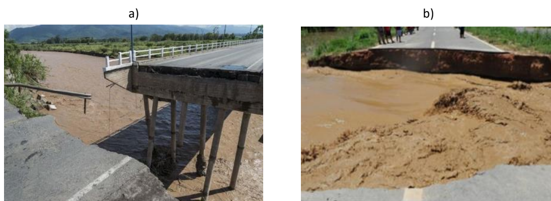
Figure 6.19. Flooding damage in Argentina; a) failure of a bridge over Lules river in 2015, [72]; b) failure of road infrastructure, Santa Victoria Este, 2018, [73].
