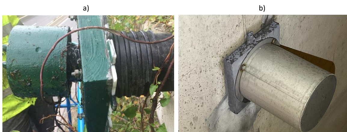
Figure 5.2 Mitigation of consequences of an anchor failure in Austria; a) an anchor failure; b) an anchor head protection; ©ASFINAG.
