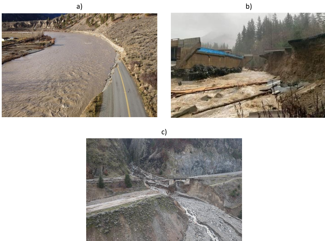
Figure 6.8 Damage to infrastructure due to the atmospheric river event ; a) a major washout on Highway 8; b) the collapse of Bottletop Bridge on Highway 5; c) destroyed rail and road lines at the Tank Hill underpass; ©BCMoTI.
