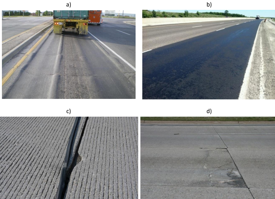
Figure 3.3 Common pavement damage due to temperature changes. a) asphalt surface rutting; b) asphalt surface flushing; c) loss of pre-formed neoprene joint sealing (a rapid cooling event); d) spalling of concrete slabs (thermal expansion); ©Hein, D.
