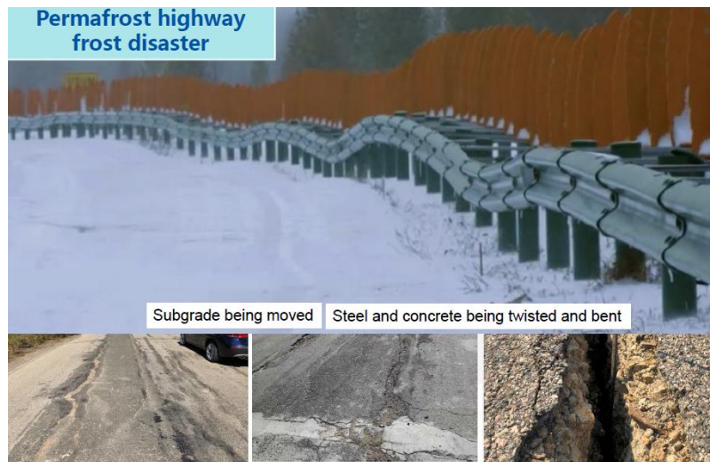
Fig. 3 – Highway problems due to subgrade movement
