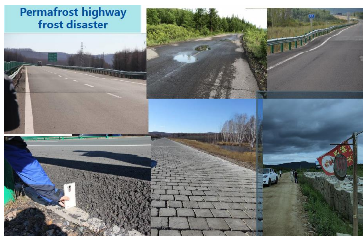
Fig. 4 – Highway problems due to frozen soil melting
