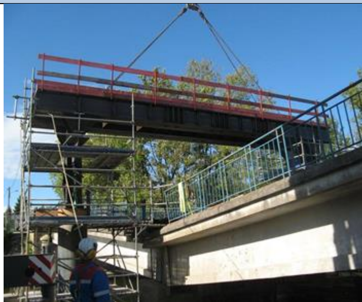
#06 France (2): Strong flood due to the storm JOACHIM caused the subsidence of pier P1 by 2m
