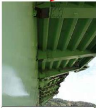
Deformation and Fracture of Bracket
