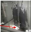
Deformation and Fracture of Web
