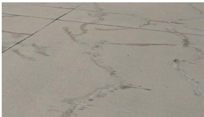
Figure 77: Shrinkage cracks, right after application of the repair liquid (2020)
