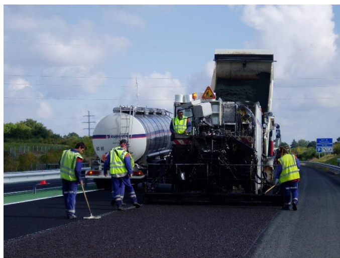
Figure 23: A 87 treatment application
