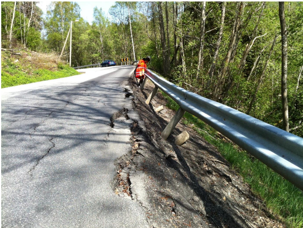
Figure 52: Longitudinal cracking and damage at the edges of the road due to settlements [4]
