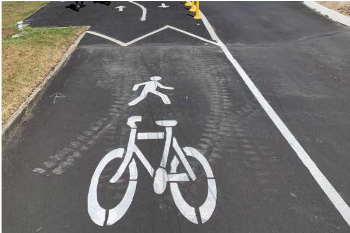
Example of shared bicycle lane. Sharing with pedestrians entails a risk of collision.
