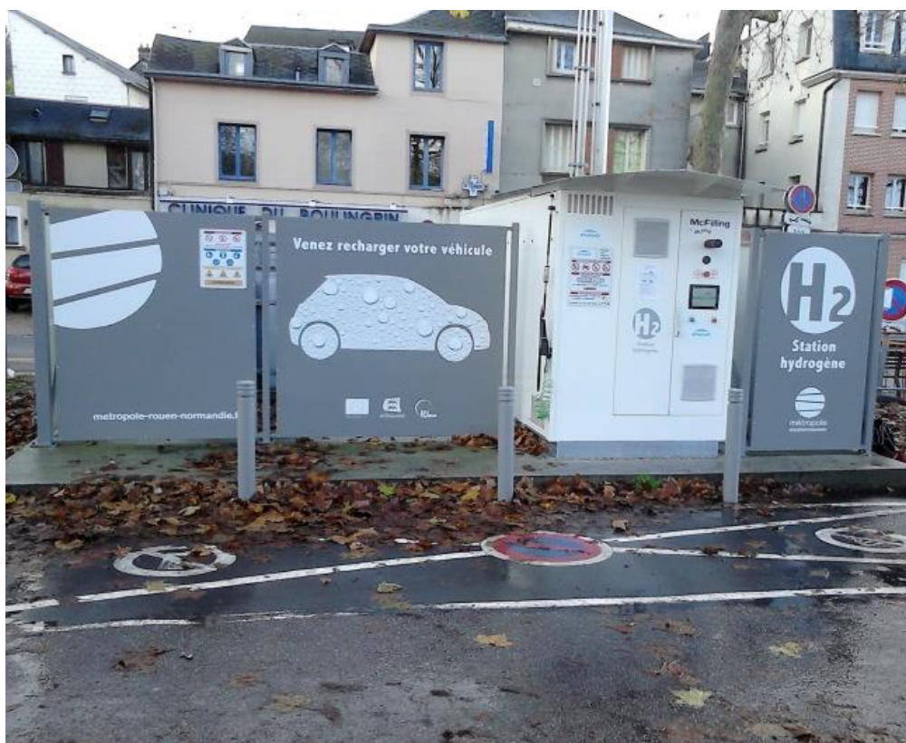
Copyright: INEA The hydrogen refuelling station in Rouen
