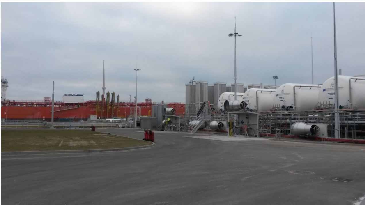
LNG bunkering facility and on shore station in the Port of Klaipeda (Source: INEA)
