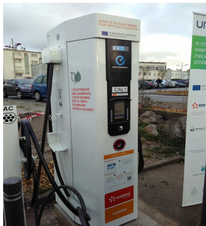
Fast-charging station deployed in the UNIT-E project (Source: INEA)
