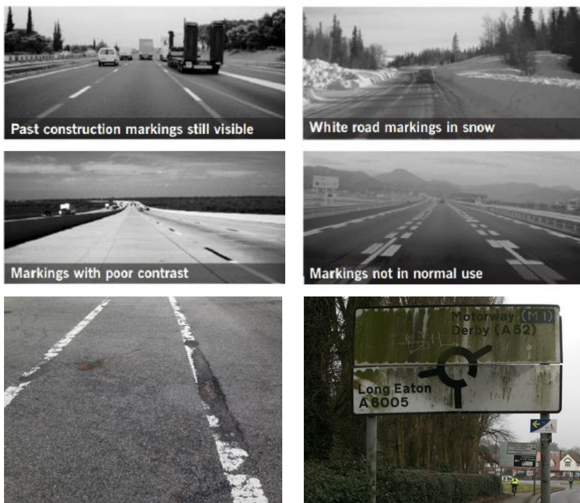
Figure 17 : Examples of pavement marking and road sign maintenance issues [14]
