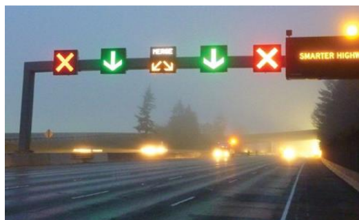
Figure 7 : Lane Use Management Sign (LUMS)
