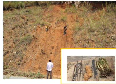
Figure 9: Site preparation and grass planting tools
