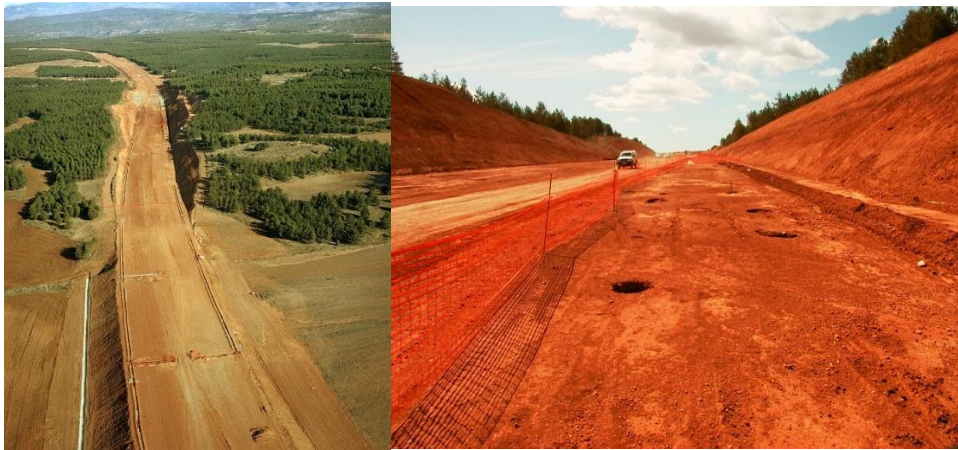
Fig.1 (left) Aerial view of the cuttings affected by the phenomenon Fig. 2 (right) Sink holes observed in the bottom of a cutting
