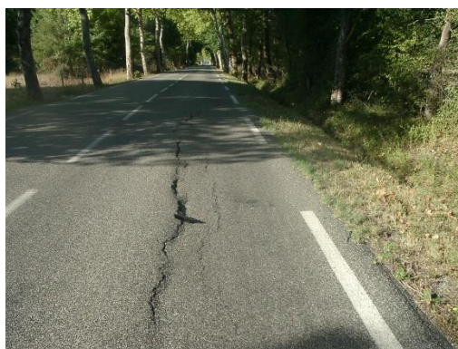
Figure 19: Example of damages in the south of France.
