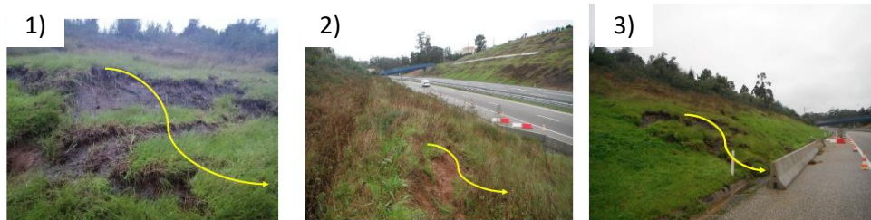
Figure 1 – Damage: Photos: 1, 2 and 3)
